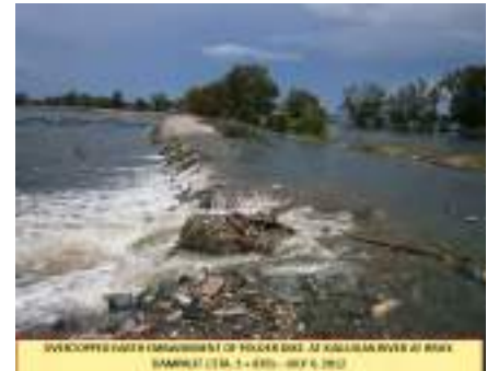
Overtopped earth embankment at Kailugan River at Barangay Dampalit, Malabon City
