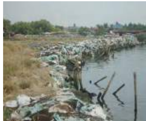
Portion of the damaged polder dike
