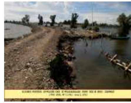
Scoured portion of Polder Dike at Pinagkabalian River side at Brgy. Dampalit (Tide level at 2.2 m – July 5, 2012)
